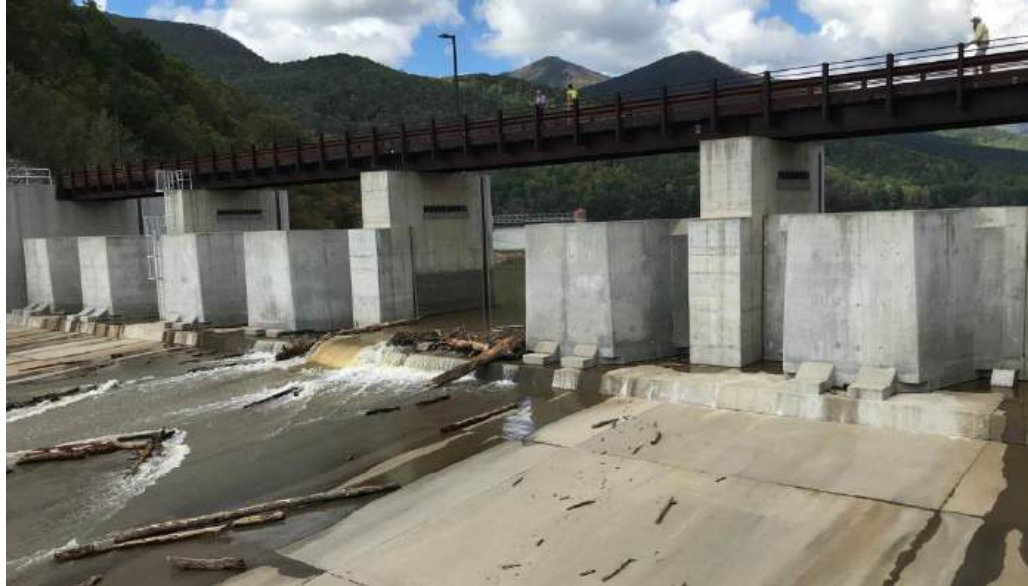
North Fork Reservoir Auxiliary Spillway on October 2 nd – fuse gate spillway system functioned as designed.
