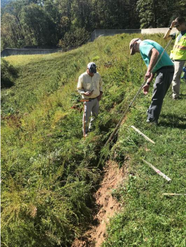
Measuring a surficial crack at the top of Bee Tree Dam on October 2 nd .
